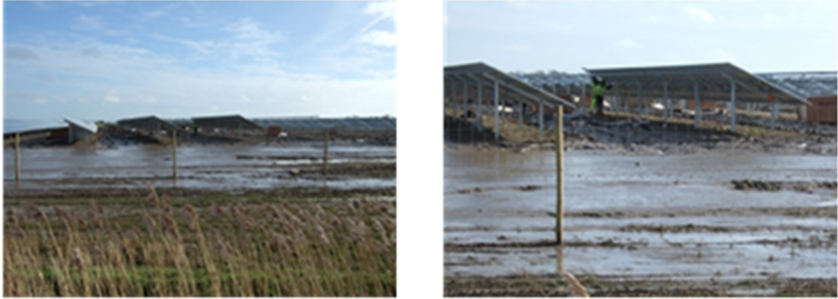
Figure 2 Solar installation at New Romney showing the effects compaction (associated with Solar Panel installation) has on surface water
