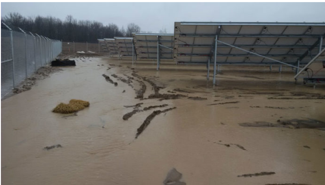
Turbid runoff from a solar project during construction.
